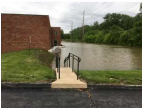
Existing buildings along S. River Road routinely flood, most recently in 2017 and 2019.
